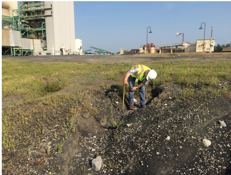
Photograph No. 2 Pond 004 Minor rutting and erosion in upstream slope
