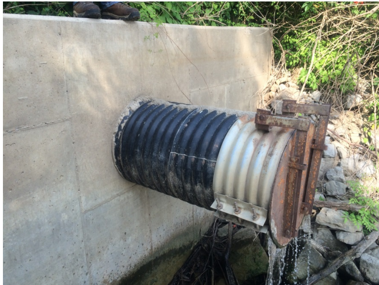
Photograph No. 12 Pond 004 Discharge pipe to Mississippi River with backflow preventer
