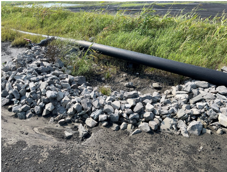
Photograph No. 16 UWL Catch basin and associated stormwater pipe at top of Phase I
