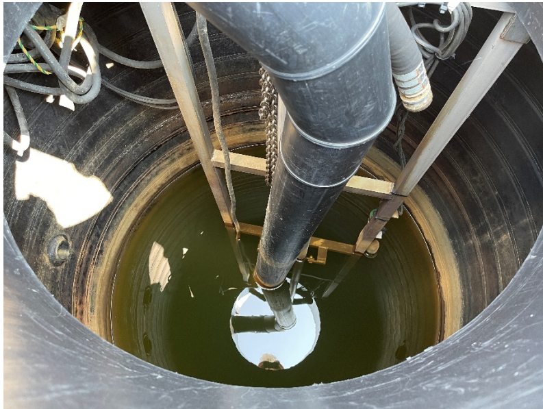
Photograph No. 32 UWL Leachate Pond loadout structure manhole
