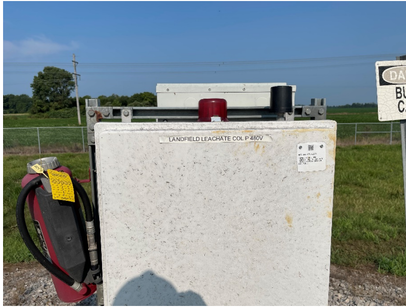
Photograph No. 11 UWL Electrical control box related to landfill leachate pump
