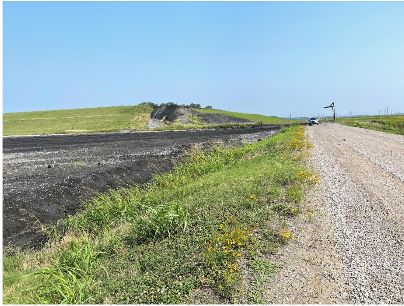
Photograph No. 23 UWL Phase III eastern perimeter berm/road Phase I in background
