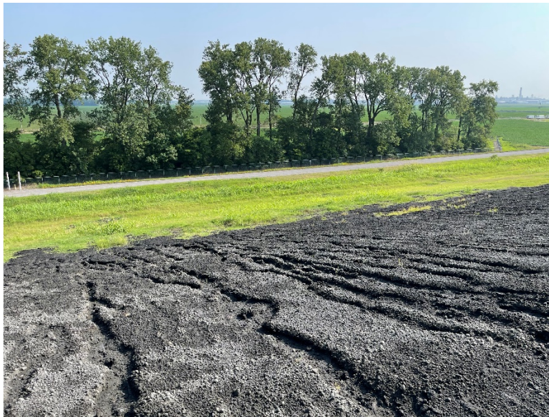
Photograph No. 18 UWL Erosion in exposed CCR on top of northern face of Phase I
