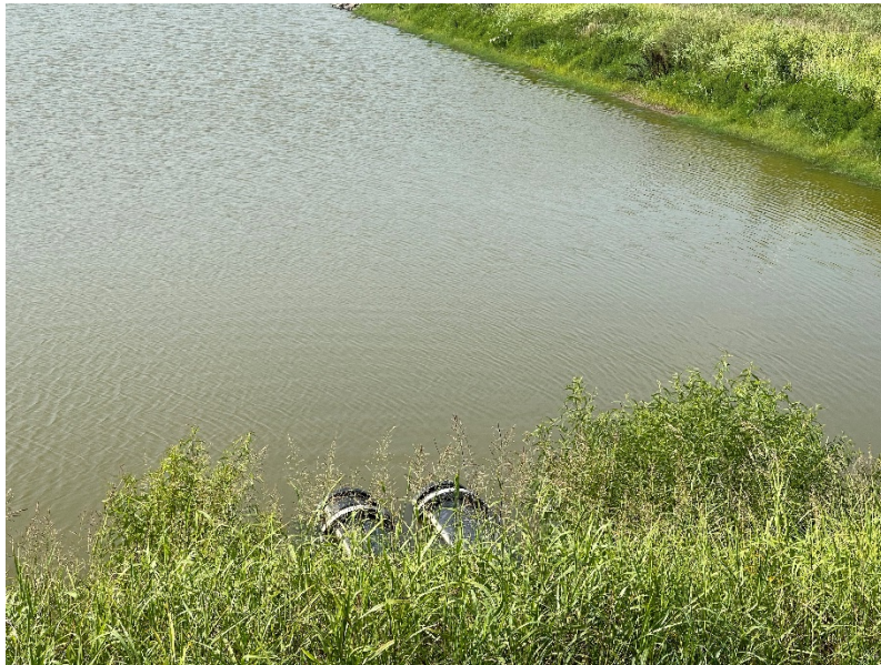
Photograph No. 22 UWL Sedimentation ponds equalization pipes
