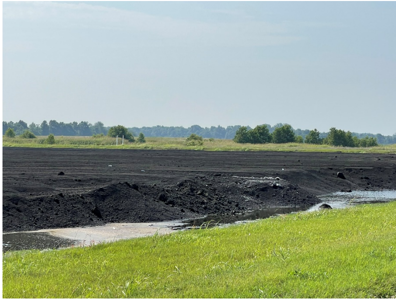
Photograph No. 29 UWL Placement of CCR in Phase III Upstream slope of west berm in foreground
